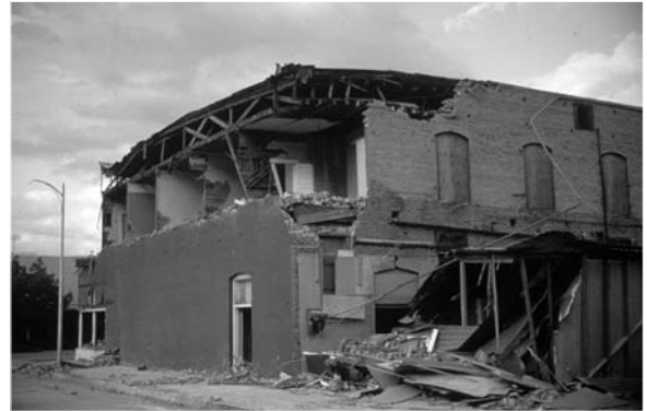
▲ 11.2 Collapse of exterior wall. 1983 Coalinga, California earthquake (Reproduced with permission from R.B. Shephard).
