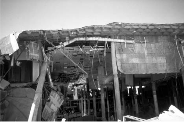
▲ 5.37 Two suspended waffle slabs have collapsed. Retail store. 1994 Northridge earthquake, California. (Bertero, V.V., Courtesy of the National Information Service for Earthquake Engineering, EERC, University of California, Berkeley).
