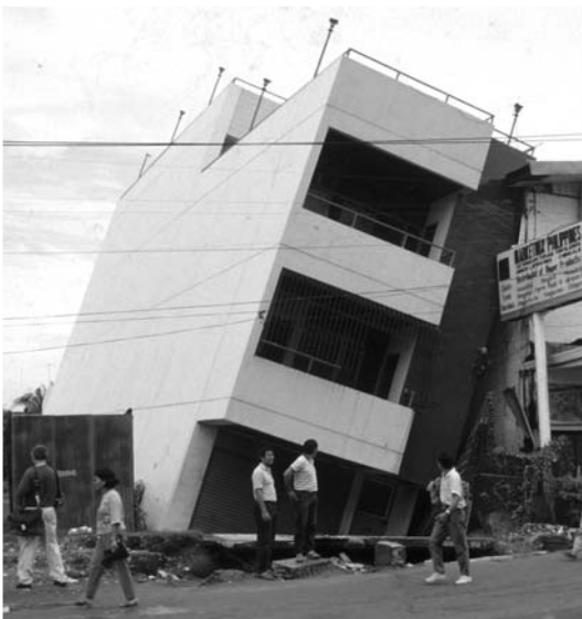
▲ 7.3 A building after liquefaction. Dagupan City, 1990 Philippines earthquake. (Reproduced with permission from David C. Hopkins).
