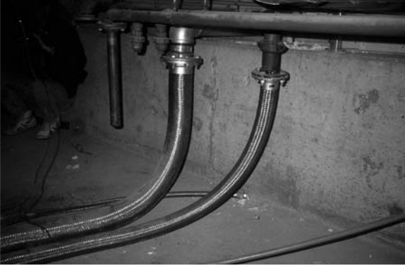
▲ 14.10 Flexible services pipes. Seismically isolated office building, Wellington.
