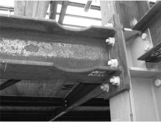
▲ 5.48 Intentional weakening of a moment frame beam to form a structural fuse. The fuse region is weaker than any other structural member or connection. The wood flooring is unusual, but appropriate for this hotel built above an existing concrete parking building. Wellington.
