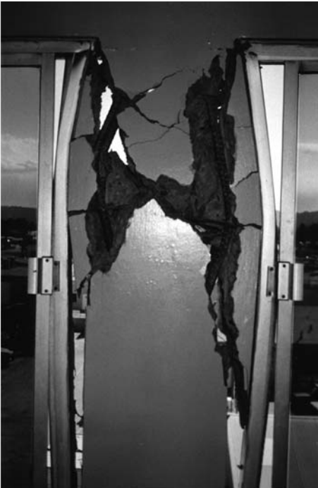
▲ 3.13 Brittle reinforced concrete column shear failure. Los Angeles, 1994 Northridge earthquake. (Reproduced with permission from A.B. King).
