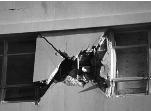
▲ 9.12 Typical short column damage. 1994 Northridge, California earthquake. (Reproduced with permission from Andrew B. King).
