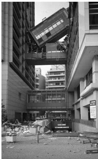
▲ 8.30 Collapsed bridge formerly spanning between two buildings. 1995 Kobe, Japan earthquake. (Reproduced with permission from US National Geographic Data Center. Dr. R. Hutchison, photographer).
