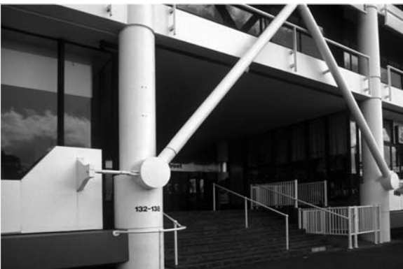
▲ 17.2 A steel damper in the form of a horizontal tapered cantilever on a building perimeter. Office building, Auckland.
