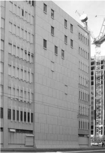
▲ 5.8 A reinforced concrete shear wall strengthens an existing building. Note how the number of penetrations per storey increases with height. Telephone exchange, Wellington.
