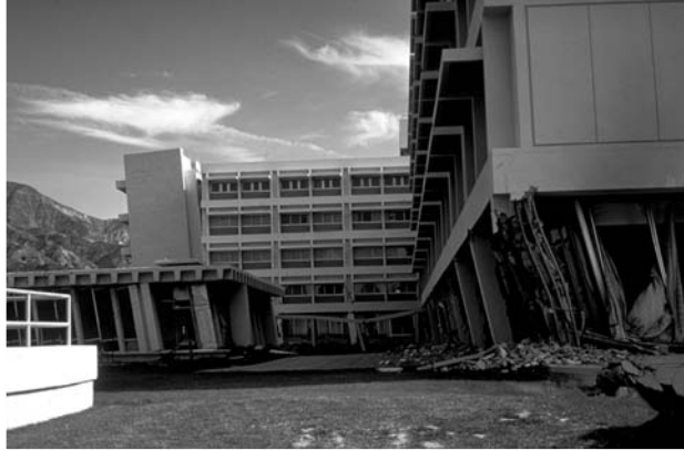
▲ 3.4 Damage to the Olive View hospital. 1971 San Fernando, California earthquake. (Reproduced with permission from Bertero, V. V. Courtesy of the National Information Service for Earthquake Engineering, EERC, University of California, Berkeley).
