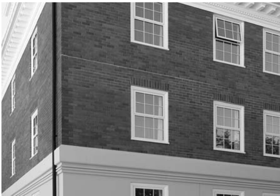
▲ 11.6 Veneer on a multi-storey wood framed building. Each storey-height of veneer is supported on a steel angle bolted to framing. Hotel, Tongariro National Park, New Zealand.
