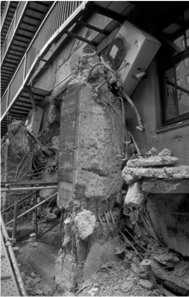
▲ 12.4 A damaged reinforced concrete building, 1995 Kobe, Japan earthquake. (Reproduced with permission from Adam Crewe).
