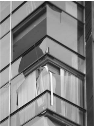
▲ 11.16 Damage to corner windows. Mexico City, 1985 Mexico earthquake. (Reproduced with permission from David C. Hopkins).
