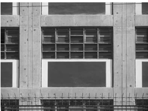
▲ 10.16 A separated partial-height infill in a moment frame. Due to the low height of the infill its out-of-plane inertia forces can be resisted by two small reinforced concrete columns. Office building, Plisco, Peru. (Reproduced with permission from Darrin Bell).
