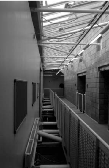
▲ 4.13 Horizontal forces from light-weight construction to the left are transferred through roof and first floor braced diaphragms to concrete masonry shear walls. Educational building, London.
