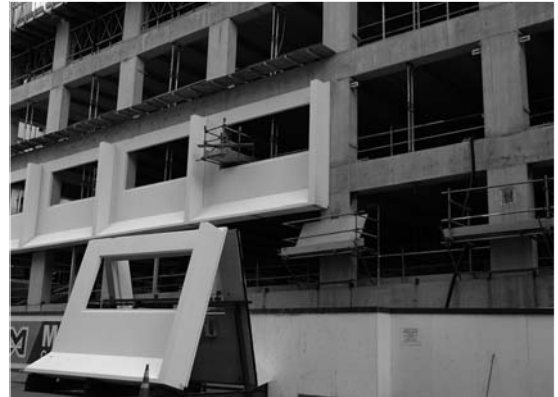
▲ 11.8 Precast panels attached to a reinforced concrete frame building. Note the connections near the tops of columns and the plane of horizontal separation between panels below the beam soffit. Office building, Wellington.
