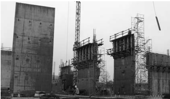
▲ 5.7 Free-standing shear walls prior to incorporation into surrounding structure highlight their vulnerability to out-of-plane forces. University building, Vancouver.
