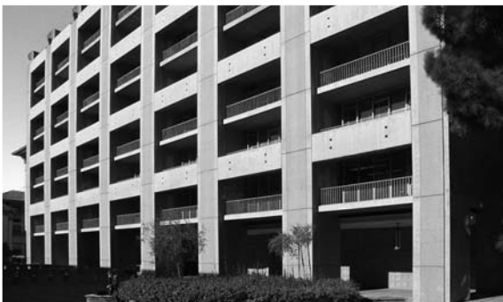
▲ 12.17 New exterior columns and beams form a double-height moment mega-frame, Berkeley, California.
