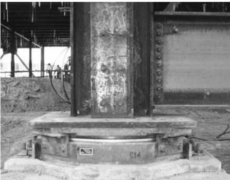
▲ 14.5 A Friction Pendulum™ bearing at the base of a column. The temporary locking brackets are yet to be removed. (Reproduced with permission. © Skidmore, Owings & Merrill, LLP).
