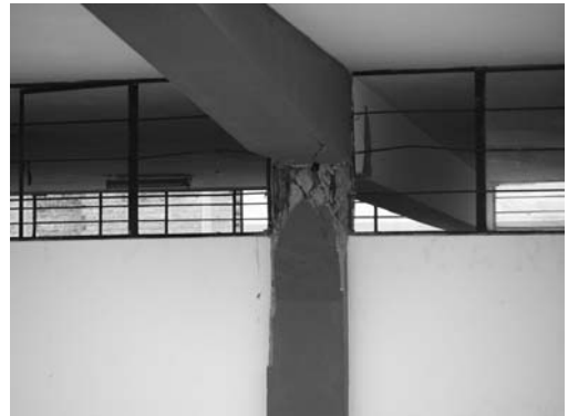
▲ 9.13 Short column failure. 2007 Pisco, Peru earthquake. (Reproduced with permission from Darrin Bell).
