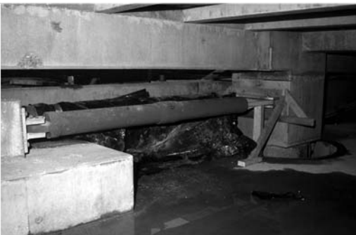
▲ 14.18 A lead-extrusion damper bolted to the foundations (left) and to the isolated superstructure (right). Police Station, Wellington.
