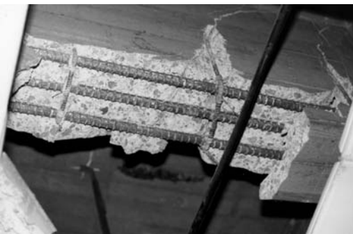
▲ 5.46 Poor example of a beam plastic hinge. The column is to the left. Mexico City, 1985 Mexico earthquake. (Reproduced with permission from R.B. Shephard).
