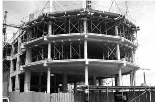
▲ 6.9 Slender gravity-only columns in the foreground with larger moment frame columns behind. Office building, Wellington.
