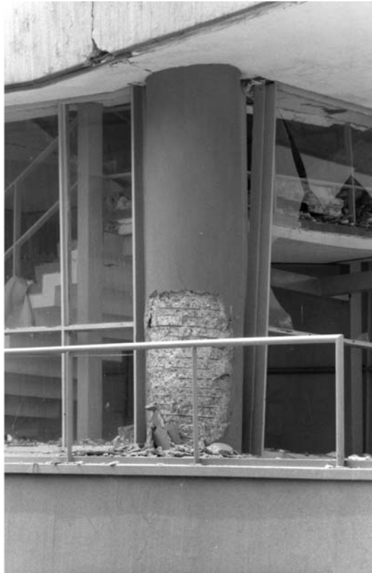
▲ 3.15 A column plastic hinge. Closely-spaced spiral ties confine the column core. Cover concrete has spalled off. Mexico City, 1985 Mexico earthquake. (Reproduced with permission from R.B. Shephard).
