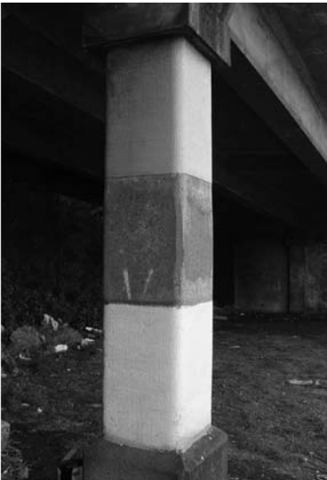
▲ 17.4 High strength fibre composite material wraps and confines potential column plastic hinge areas. Wellington.
