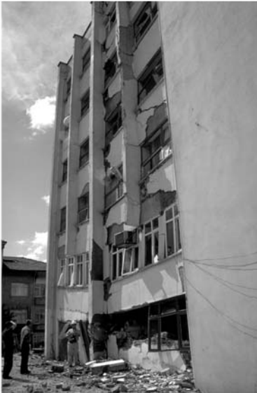
▲ 7.7 Foundation settlement of up to 500mm contributed to the building damage. 1999, Izmit, Turkey earthquake. (Sezen, H. Courtesy of the National Information Service for Earthquake Engineering, EERC, University of California, Berkeley).
