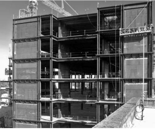
▲ 5.10 Steel shear walls during construction. Hospital, Portland, Oregon. (Reproduced with permission from KPFF).
