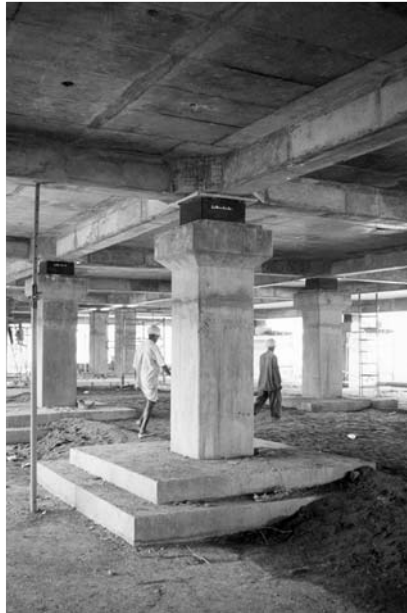
▲ 14.8 Lead-rubber bearings on cantilever reinforced concrete columns. Bhuj Hospital, India (Reproduced with permission from Adam Thornton).
