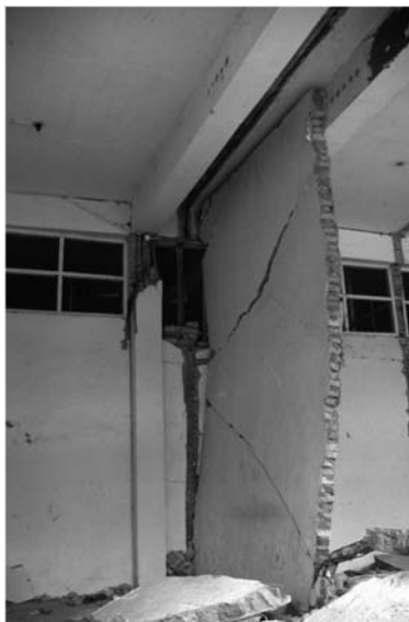
▲ 10.13 Partial out-of-plane collapse of an unreinforced masonry infill wall. Commercial building, Tarutung, Indonesia, 1987 Sumatra earthquake.
