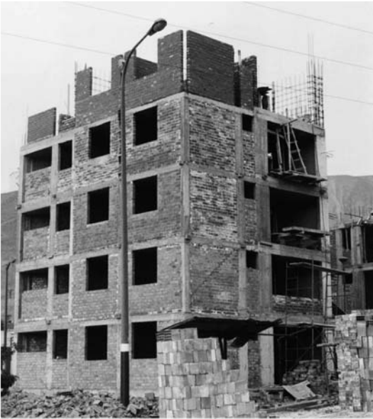
▲ 5.16 Confined masonry construction. Columns and beams are cast after laying the walls. Only walls without large penetrations and are continuous up the height of the building act as shear walls. Lima. (Reproduced with permission from Ángel San Bartolomé)
