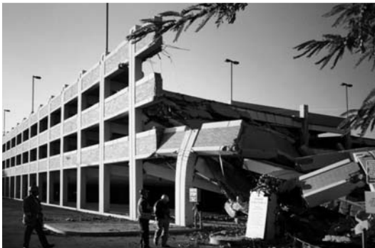
▲ 3.2 Partial collapse of a car parking garage, Los Angeles. 1994 Northridge, California earthquake. (Reproduced with permission from A.B. King)
