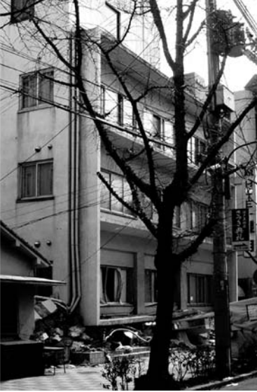
▲ 9.1 Soft storey ground floor collapse of a four-storey building. 1995 Kobe earthquake. (Bertero, V.V. Courtesy of the National Information Service for Earthquake Engineering, EERC, University of California, Berkeley).
