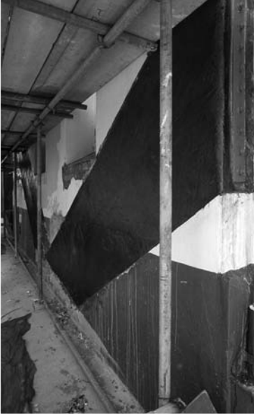
▲ 14.25 A carbon fibre strip glued onto an unreinforced masonry wall to increase its shear strength. Hotel, Wellington.
