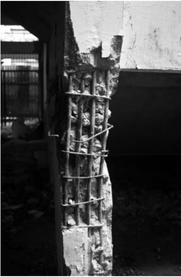
▲ 16.7 Incorrectly bent column ties led to this column almost collapsing. 1987 Tarutung, Indonesia earthquake.
