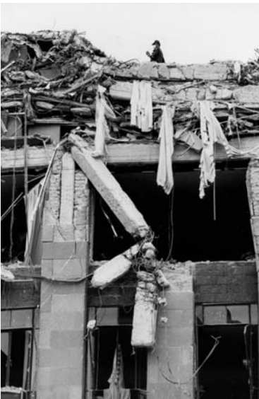
▲ 5.45 A collapsed building with weak columns and strong beams. Ironically the architect enlarged the columns with non-structural masonry. Mexico City, 1985 Mexico earthquake. (Reproduced with permission from R.B. Shephard).
