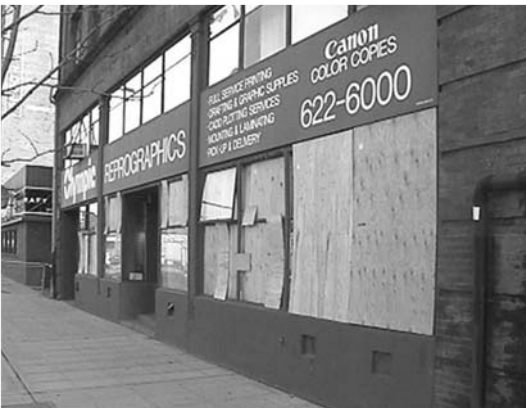
▲ 3.7 Plywood sheets cover broken windows after the small 2001 Nisqually Earthquake, near Seattle. (Reproduced with permission from Graeme Beattie).
