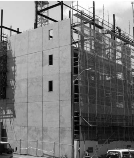
▲ 5.12 A shear wall formed from numerous precast panels strongly connected vertically and horizontally. Apartment building, Wellington.
