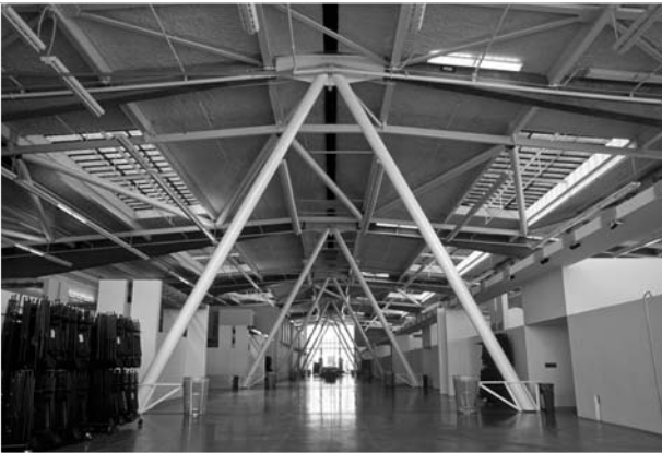
▲ 17.1 Seismic braces define the main circulation route of this retrofitted building. Educational building, San Francisco.
