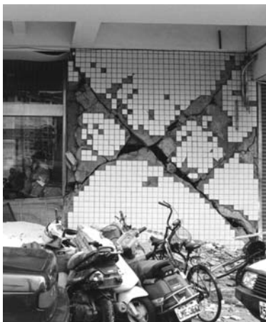
▲ 10.5 Typical infill wall diagonal crack pattern. 1999 Chi-chi, Taiwan earthquake. (Reproduced with permission from Geoff Sidwell).
