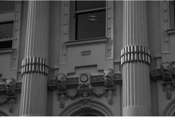
▲ 11.19 Weakly attached unreinforced columns are tied back at first floor level with stainless steel ties and vertical bearing rods. Restaurant, Wellington.
