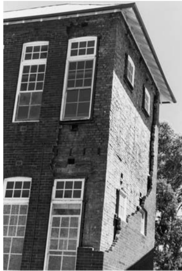
▲ 11.4 Damage to brick veneer due to corroded veneer ties. 1989 Newcastle, Australia earthquake. (Reproduced with permission from R.B. Shephard).
