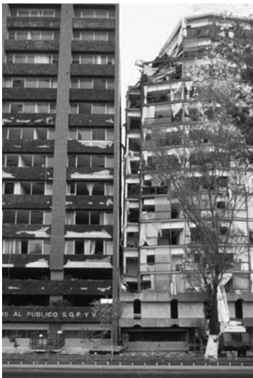
▲ 8.23 Pounding damage during the 1985 Mexico City earthquake. (Reproduced with permission from David C. Hopkins).
