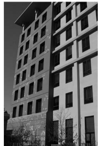
▲ 12.18 A retrofit solution consisting of exterior moment frames. The surface markings identify remedial work to surface coatings, Berkeley, California.
