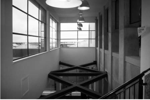
▲ 17.7 A steel cross-braced diaphragm at first floor level. Library, Palmerston North, New Zealand.
