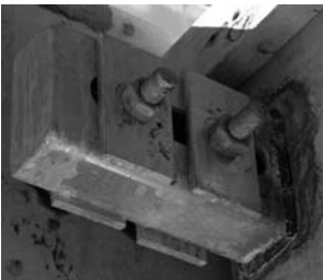
▲ 11.9 Slotted steel connection welded to a plate cast into the column (a) and the completed detail allowing movement (b).
