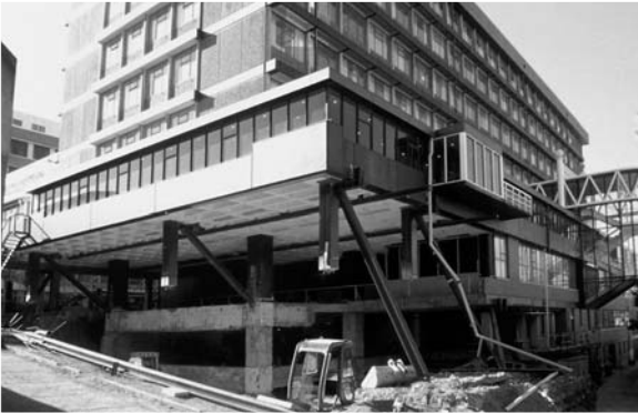
▲ 14.13 An area of the podium is propped while excavation is completed prior to installation of lead-rubber bearings. Library, Wellington.
