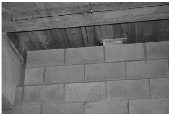
▲ 10.12 A reinforced masonry infill wall separated from surrounding structure. Note the horizontal and vertical gap (to beam) and a galvanized steel bracket resisting out-of-plane forces yet allowing in-plane movement. Office building, Wellington.
