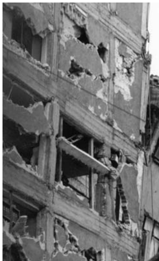
▲ 10.6 Damage to the tops of several columns due to infill wall compressive strut action. Mexico City, 1985 Mexico earthquake. (Reproduced with permission from R.B. Shephard).
