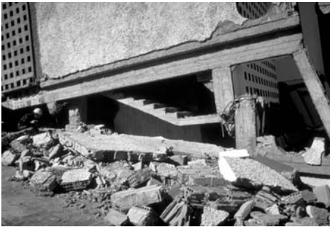
▲ 9.17 Ground floor damage caused by a discontinuous wall. 1980 El Asnam, Algeria earthquake. (Bertero, V.V. Courtesy of the National Information Service for Earthquake Engineering, EERC, University of California, Berkeley).
