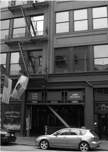
▲ 12.1 Braced retrofit structure poorly integrated with the existing architecture, San Francisco.
