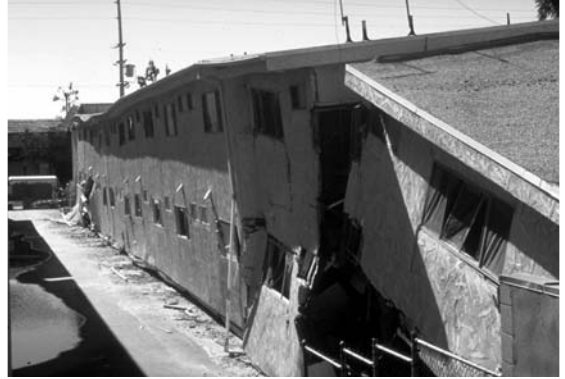
▲ 9.2 A soft storey ground floor has disappeared in this three-storey apartment block. 1994 Northridge, California earthquake. (Reitherman, R.K. Courtesy of the National Information Service for Earthquake Engineering, EERC, University of California, Berkeley).
