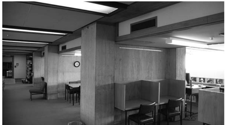
▲ 17.6 Reinforced concrete shear walls where the wall chords are differentiated from the webs. Educational building, Wellington.
