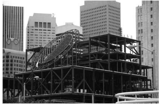
▲ 6.21 Braced steel structure of the San Francisco Museum of Modern Art during construction.
