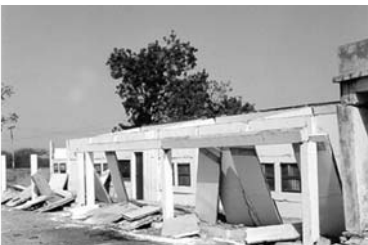
▲ 16.1 A damaged precast concrete school building due to failure of roof panel connections. 2001 Bhuj, India earthquake. (Reproduced with permission from IIT Bombay Team).
