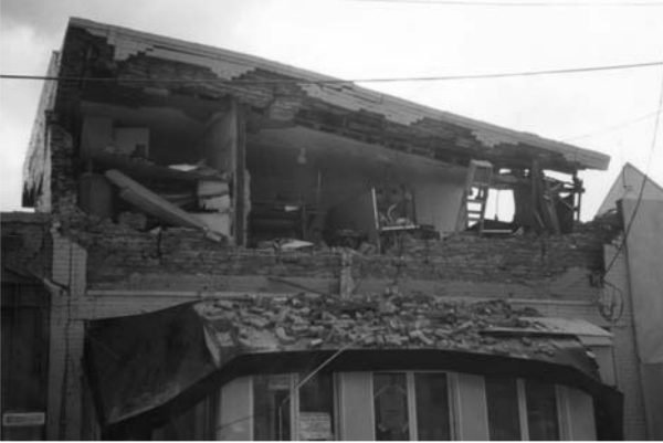
▲ 4.2 The weakness of unreinforced masonry walls and their connections prevented inertia forces being transferred safely to diaphragms at first floor and roof level. Santa Monica, 1994 Northridge earthquake.
