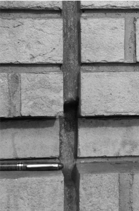
▲ 6.22 Separation joint between panels of brick masonry filled with flexible sealant. San Francisco Museum of Modern Art.
