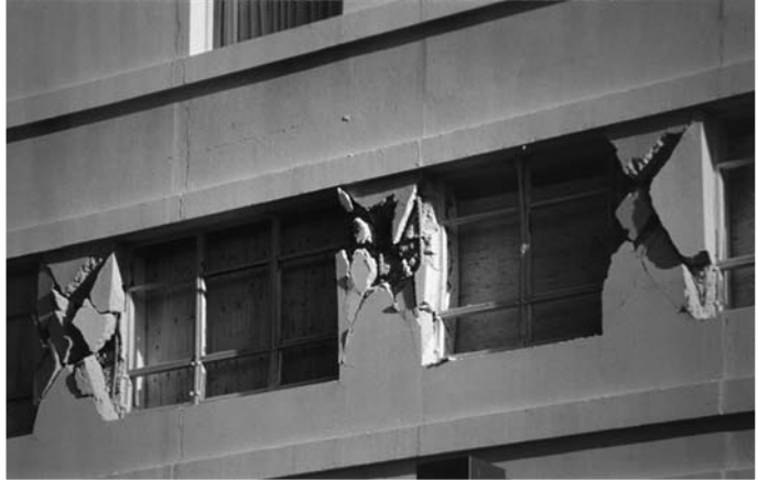
▲ 5.33 Column shear failure in a moment frame. 1994 Northridge earthquake, California. (Reproduced with permission from A.B. King)
