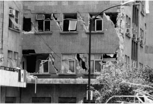
▲ 11.1 Unseparated masonry cladding damaged by the interstorey drift of a flexible internal steel frame. Mexico City, 1985 Mexico earthquake. (Reproduced with permission from R.B. Shephard).
