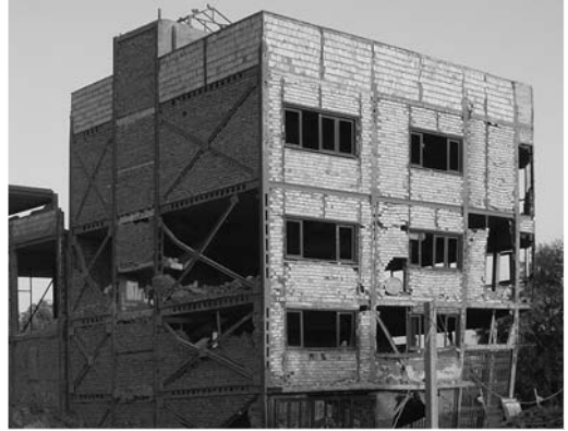
▲ 16.6 Inadequate welds caused three brace failures. Bam, 2003 Bam, Iran earthquake. (Reproduced with permission from Jitendra Bothara).
