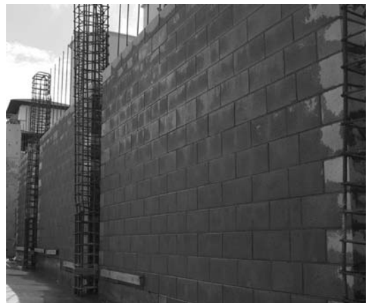
▲ 5.13 A reinforced concrete masonry wall with attached columns under construction. Horizontal reinforcing, placed every third masonry unit is not visible. Office building, Wellington.
