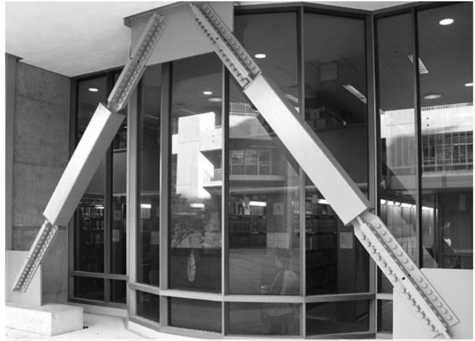
▲ 14.20 Buckling-restrained braces improve the seismic resistance of an existing building, Berkeley, California.
