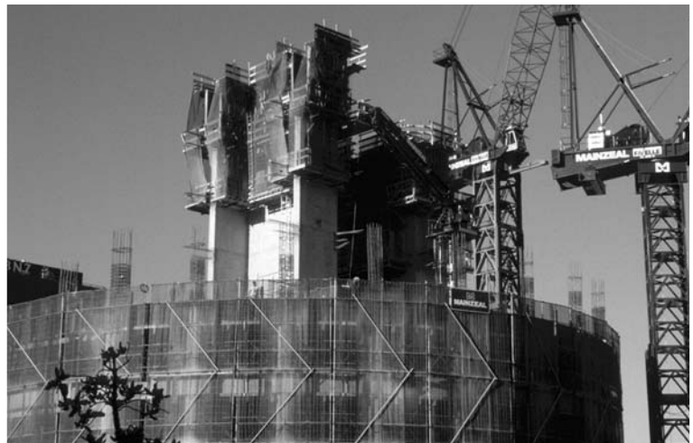
▲ 5.51 A mixed structural system. A central shear wall core with a perimeter moment frame under construction. Office building, Wellington.
