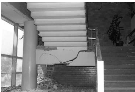
▲ 10.20 Damage to stair support structure. Mexico City, 1985 Mexico earthquake. (Reproduced with permission from R.B. Shephard).
