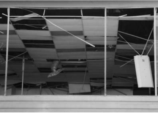
▲ 11.21 Suspended ceiling damage. 1994 Northridge, California earthquake. (Reproduced with permission from A.B. King).
