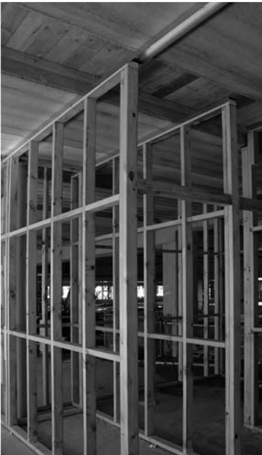
▲ 11.20 Framing for interior partition walls. The wall top plate is inserted into a sheet steel channel without being nailed to it. This detail allows relative movement in the plane of the wall between the wall and the floor above. Office building, Wellington.
