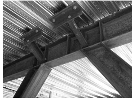
▲ 5.26 An eccentrically braced frame with stiffener plates and fly-braces to stabilize the beam bottom flange in the structural fuse region. Apartment building, Wellington.
