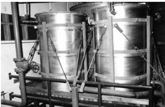
▲ 11.25 A braced roof-top water tank. Hospital, Whakatane, New Zealand.
